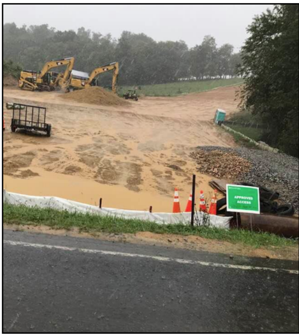
Left: sediment prepares to pour across Blue Ridge Parkway in one of 250 water quality violations on Mountain Valley Pipeline.
