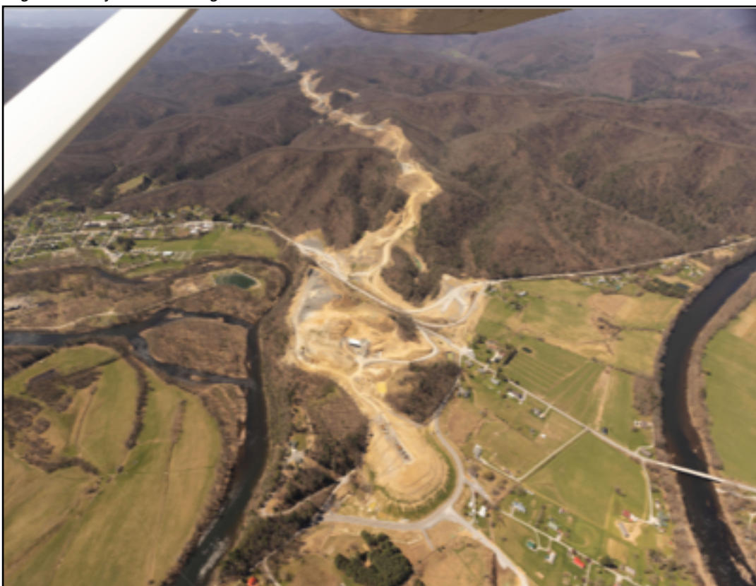
Below: Corridor H construction. Holly Meadows area looking Southwest. Photo by Mark Moody. Flight courtesy of SouthWings Volunteer Pilot Don Sutherland.
