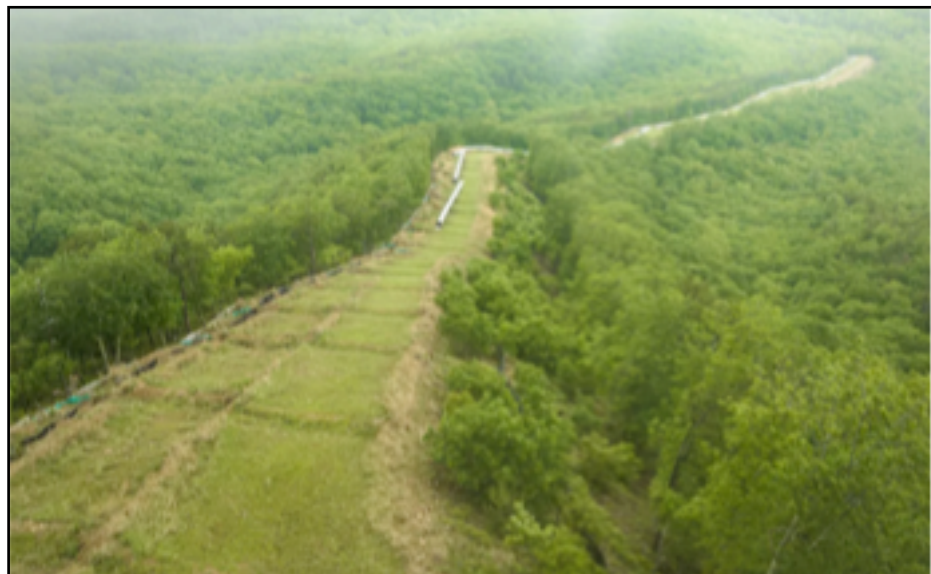
The Mountain Valley Pipeline construction site in the Jefferson National Forest, Virginia. Photo courtesy The Wilderness Society.
